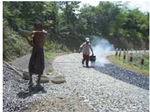
Fig. 1. Paving the road with asphalt. It is a very simple treatment on which tar is applied over pebbles. August 18, 2007.
