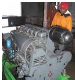
Fig. 34. The diesel generator at the power plant in Kanpetlet. Because the diesel is extremely limited, electric supply to the town is very limited (once a week, about two hours per one night).
