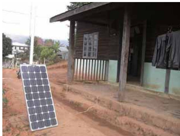
Fig. 38. A solar panel is also being used for back-up power
