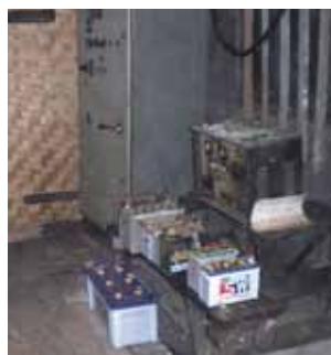
Fig. 35. Homes that have batteries bring their battery to the generator house and charge them up. It takes an entire day to charge and costs about 1,000 Kyats.
